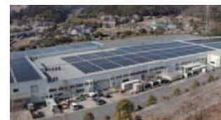
Solar panels on Osawa Plant
